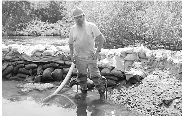
Steve Mikle pumps out water in a marshy area near the gristmill he is helping renovate.
