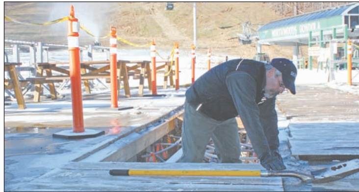
Tom Utley, a building maintenance worker and CSEA member, makes repairs to radiant heating on a wooden walkway at Gore Mountain.
