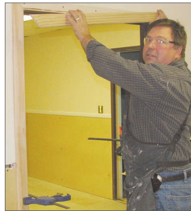
Woodworker John Parmiter replaces the trim on an office door at the town of Hempstead Department of Public Works building after it was flooded during Sandy.
