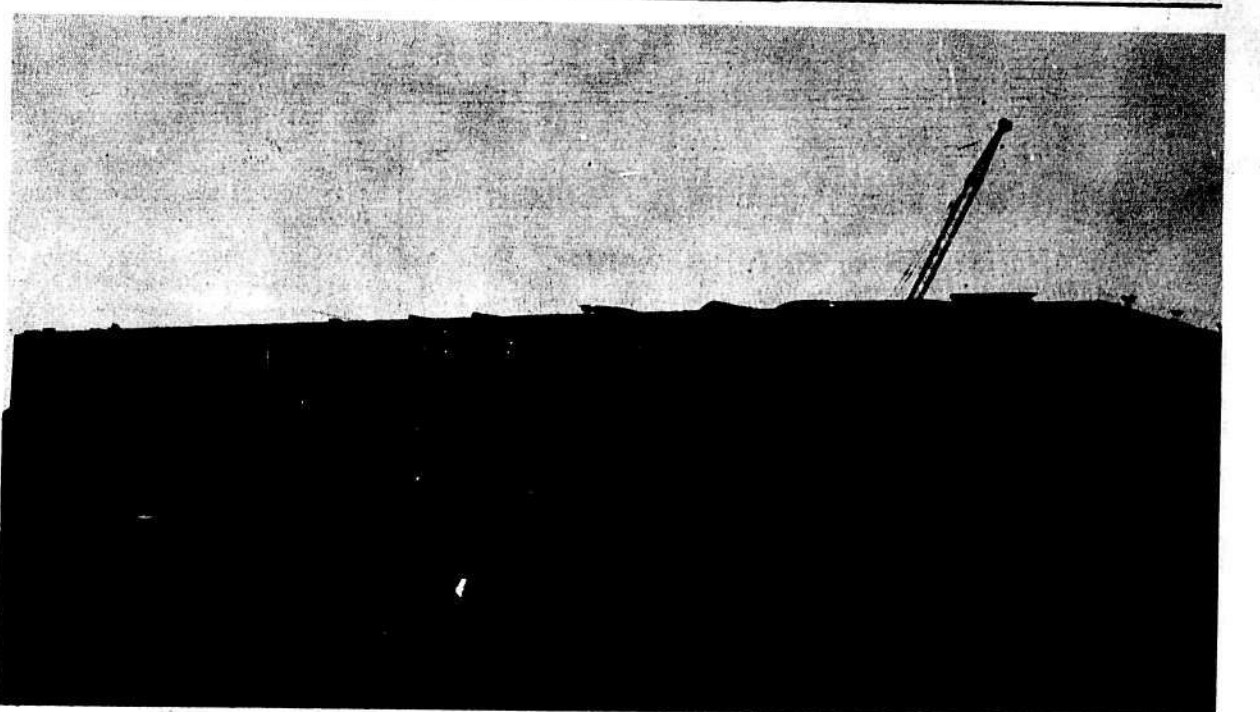
Work on the first dormitory on the new campus is progressing rapidly. Students will draw selection numbers today, to determine who the first 500 occupants of this building will be.
