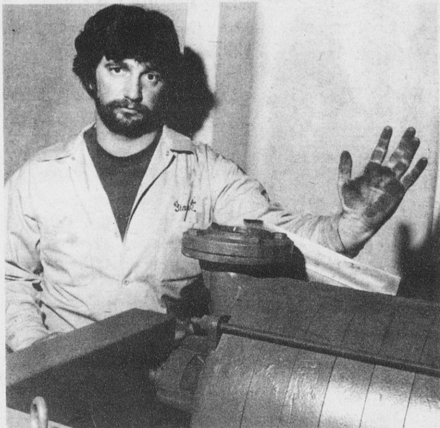
BLACK, SICKENING SOOT covers everything inside the power plant, as CSEA Shop Steward Frank Celentano, above, shows.
