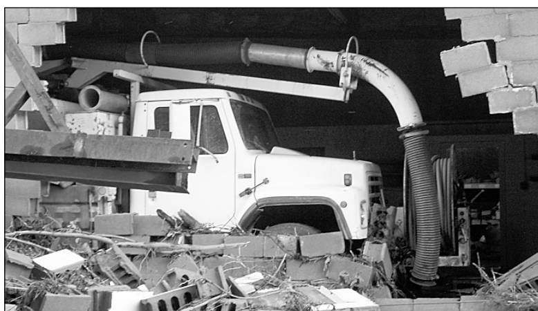
A powerful flood knocked this hole in a brick wall in a Silver Creek Department of Public Works building. The department lost all its buildings and almost all its equipment in the flooding.
