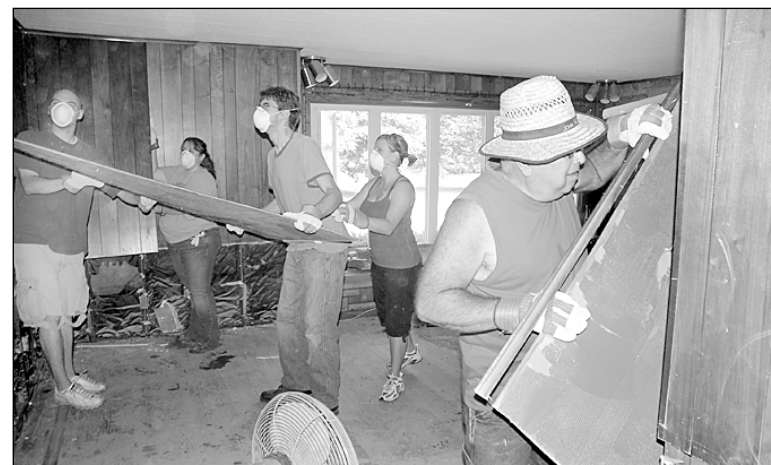
CSEA members gut a Gowanda resident's house following the flooding as part of the cleanup effort, with the volunteers removing everything right down to the studs. Photo by Albert T. McCracken Jr.
