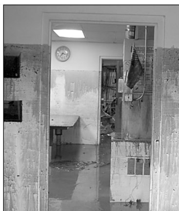
The water line remains visible inside the Silver Creek highway garage after the department's buildings and equipment were submerged in water.
