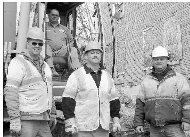
From left, demolition crew members Dave Bouchard, Bob Crews (in excavator cab), Dick Kane and Foreman Shawn Cotton.
