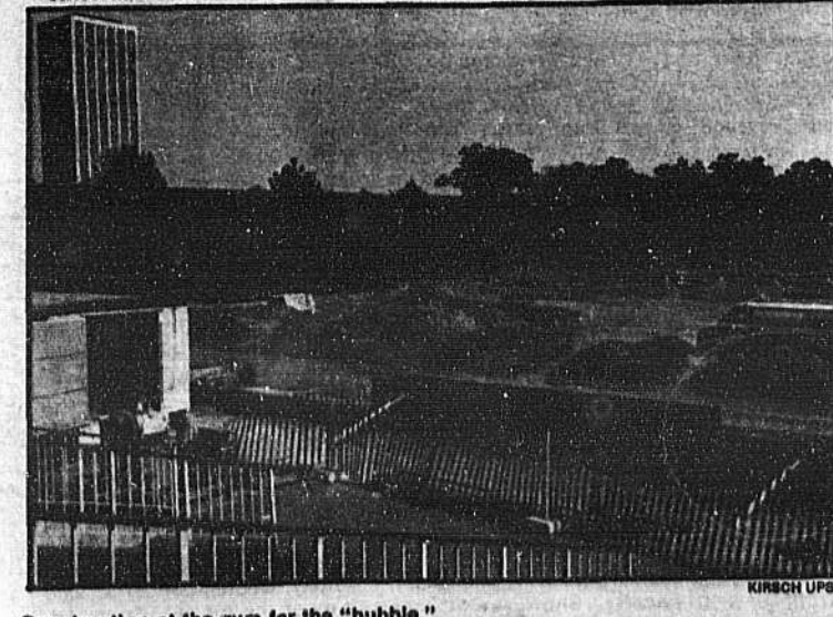
Construction at the gym for the "bubble." Four basketball and volleyball courts plus a track will be built.
