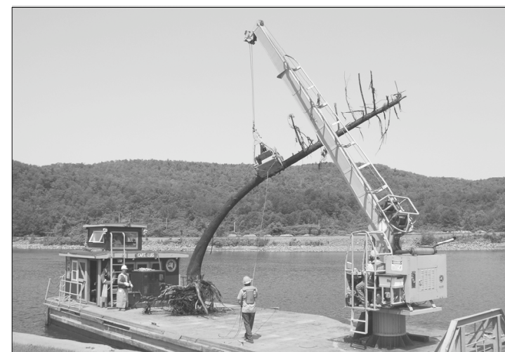
A Canal Authority scow crew removes trees and other debris from the Erie Canal. Sections of the canal from Lock 9 to 15 were affected by heavy flooding. Erosion, utility and structural damage and significant debris trapped in canal gates and lock mechanisms were to blame. From left, Canal Authority Local members Louis King, captain, Bruce Pavlus, Machinist Bob Lisco and Crane Operator Ron Klump haul a tree from Lock 13 gates.
