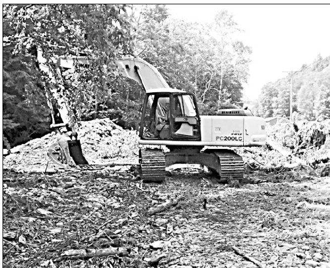
A Delaware County DPW workers clears flood debris from a ravaged County Route 16. This scene is a familiar one in the dozen counties hit by recent floods.
