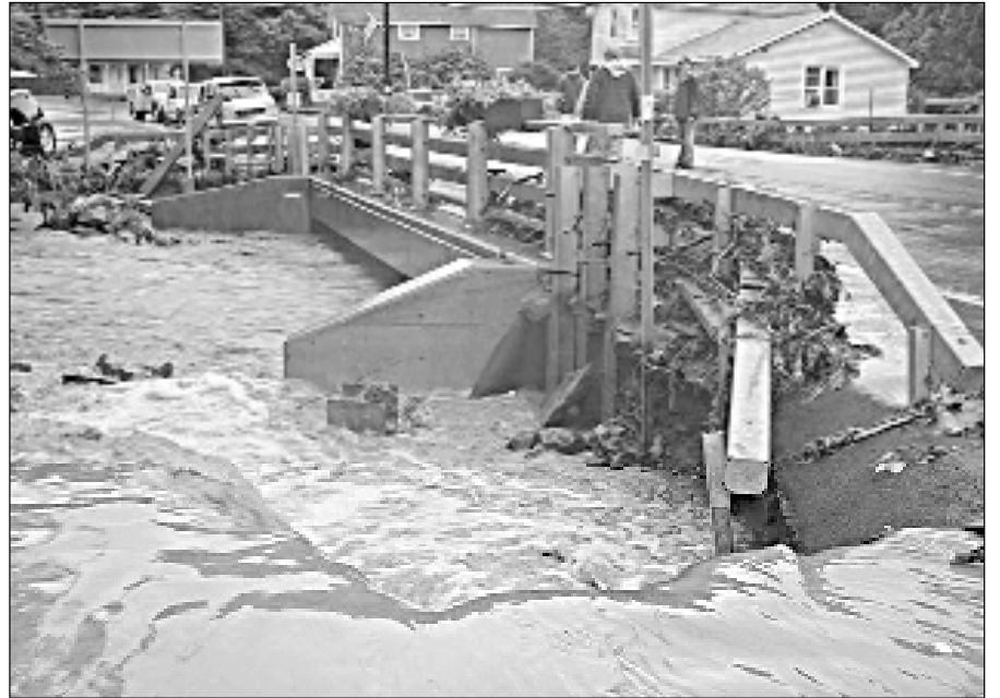
A bridge in Sullivan County is overwhelmed by flooding in this image shot by a state Department of Transportation worker.
