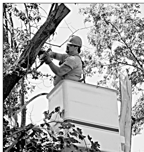
Ron Ruvo, Mount Pleasant Blue Collar Unit president and a Traffic Safety Department worker, removes tree limbs damaged in a tornado.
