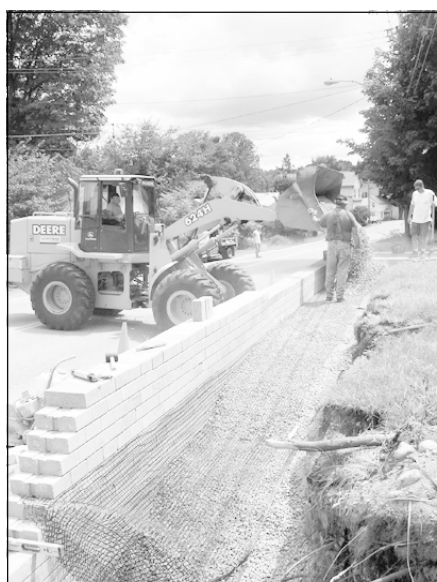
Highway workers unload gravel to backfill a new wall. From left, operating the loader, are Clarke Griffin, Howard Meade and Jason Monroe.
