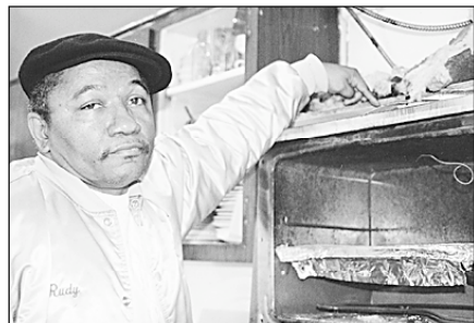
Rudy Bruce points out the damage sustained to his kitchen by an electrical fire.
