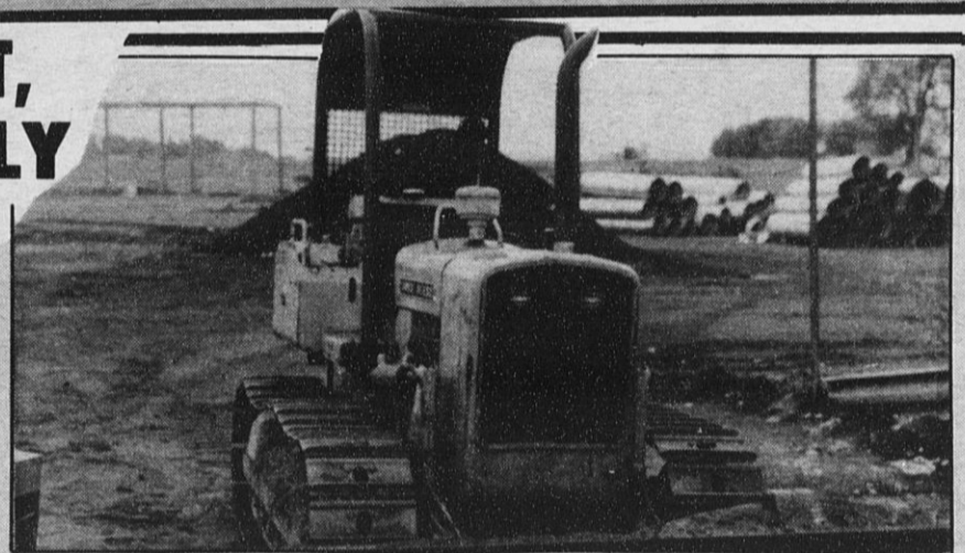
THIS WAS THE BULLDOZER that Richard Ortlieb was operating at the time he was fatally injured when pinned between the bulldozer and the underside of a bridge. CSEA officials say the roll-bars were not on the machine at the time of the mishap and could have prevented the mishap from occurring.
