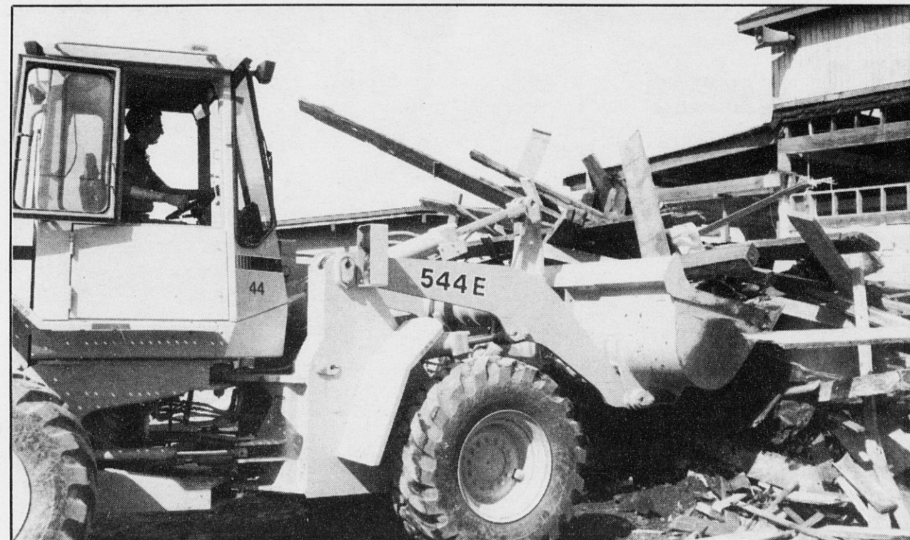
ONE OF THE HEADLINE EVENTS at this year's fair was not even on the schedule. A tornado briefly touched down, ripping the roof off this animal stable. CSEA member Mark Kolceski, a general mechanic, helps clean up the debris.
