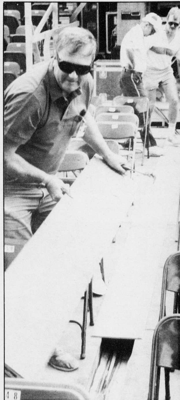
GENERAL MECHANIC JOHN RUSTON removes boards to install wiring to the grandstand's sound board. In background, General Mechanic Dan Griffin, right, gives instructions to one of many laborers working to set up next show. Ruston has worked at the fair for 21 years, Griffin for 10.
