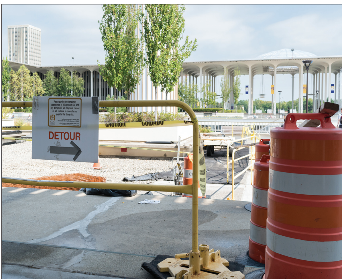
Madeline St. Amour / Albany Student Press There has been continuous construction at the university for a few years. The Campus Center construction has been ongoing since last year.
