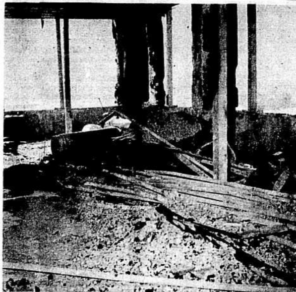
A PICTURE OF DESTRUCTION depicts the aftermath of the fire that swept the partially completed dormitory tower Thursday. The propane gas tanks amidst the rubble are blamed for the fire.
