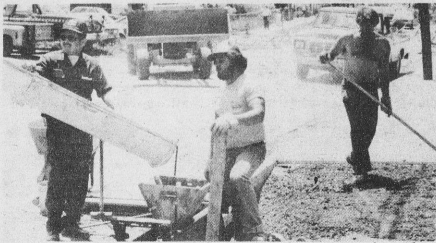
SARATOGA SPRINGS DPW CREW installs curbing as part of an urban renewal project. DPW employees augmented by temporary help are doing the work in a unique "contracting in" program that helps prevent layoffs and save public funds.
