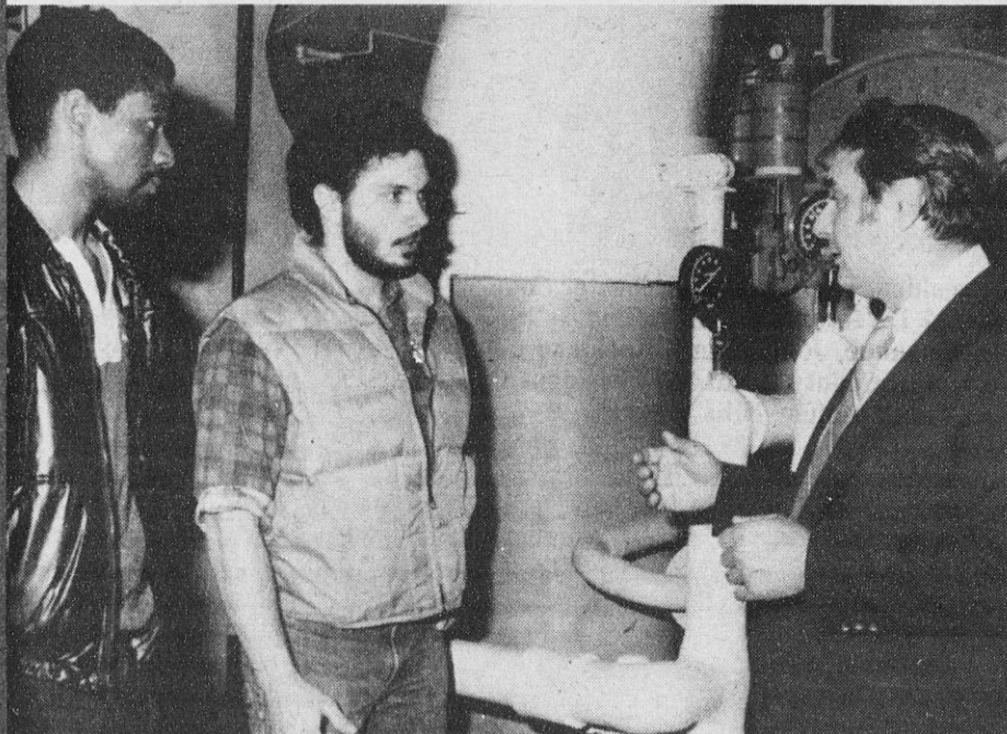
EXPLAINING THE FEATURES OF THE CHILLER FOR THE AIR CONDITIONING SYSTEM AT THE Empire State Plaza is OGS Superintendent of Plant Utilities Louis Fazzone. With him are stationary engineer trainees Clifton Rowles, left, and Joseph Franze.
