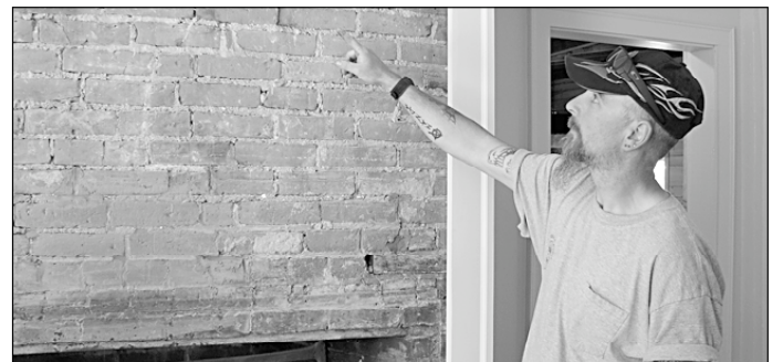
Dan Clemens shows a fireplace that was covered in plaster. Employees removed the plaster, filled holes, poured concrete and rebuilt the hearth.
