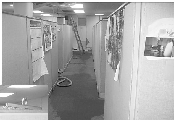
Above, Nassau's Probation Department Family Division at 1200 Old Country Road in Westbury after the office was damaged by a flood in early January. The photo at left was taken Jan. 29 to show the improvements made since the flood. Similar measures were taken at the Nassau Juvenile Detention Center on Carman Avenue which was also hit by the flood.
