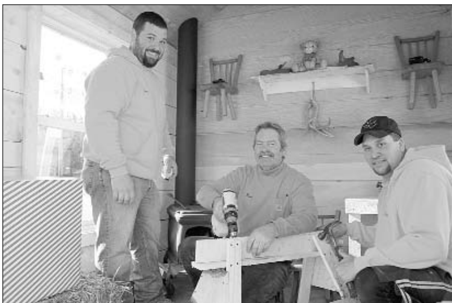
Above, Town of Patterson mechanical equipment operators, from left, Joe Tresca, Russell Goff and Jason Kinash work inside a Santa's Workshop float the Highway Department entered in the Putnam Lake Fire Department's annual holiday parade.
