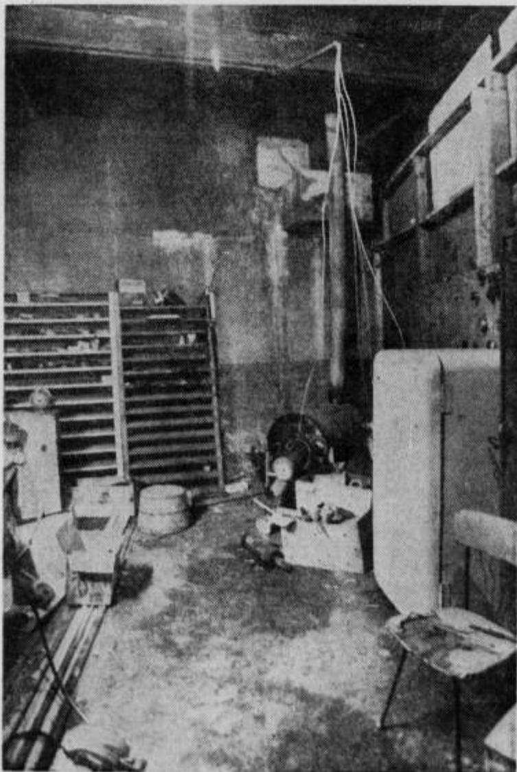
Employees repair machinery in this area of the building. The electricity supply lines are hanging, without adequate insulation from an open conduit, again in violation of every Labor Department rule or regulation.
