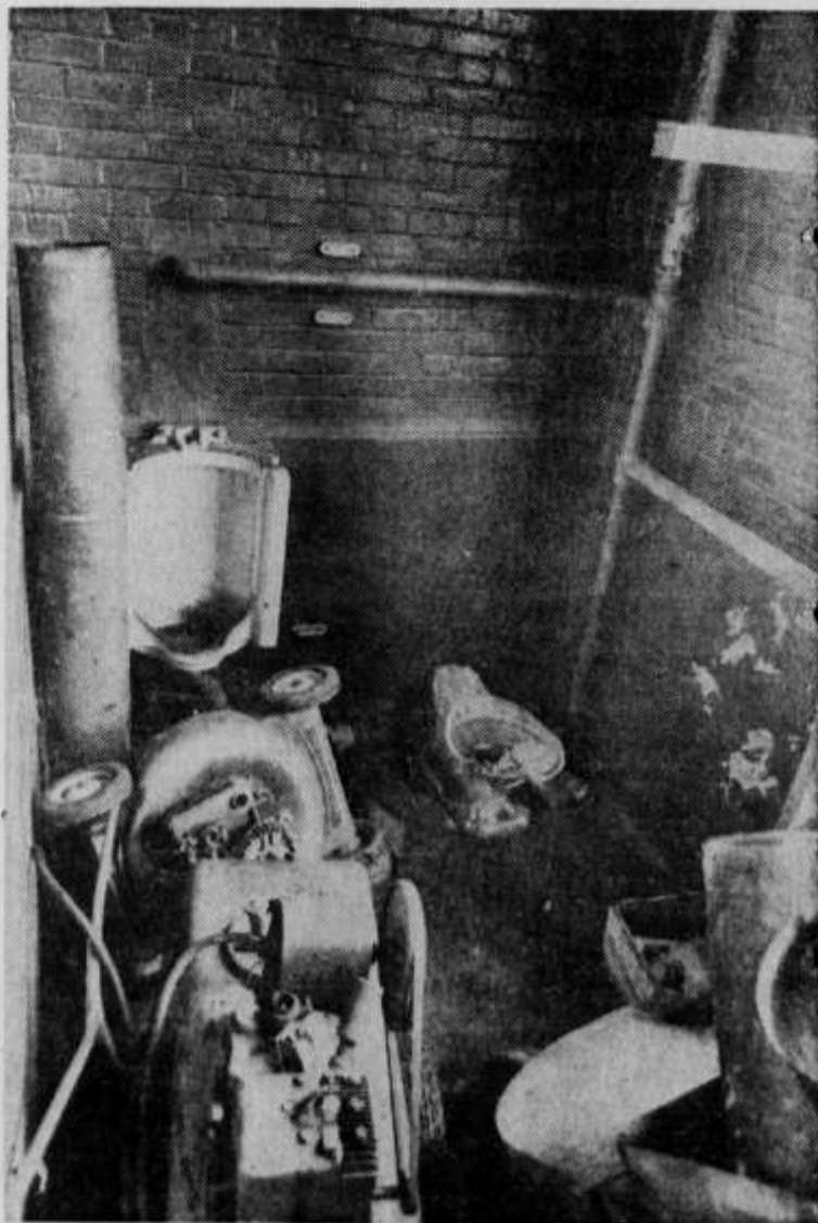
This shocking photo of the sanitary facility for male employees shows how the employees have to climb over broken plumbing supplies to enter the room.
