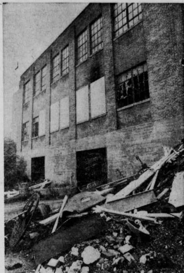
The outside of the building is littered by debris from a fire and the exit doors are open. The CSEA is complaining of the conditions which would not be tolerated in private industry.
