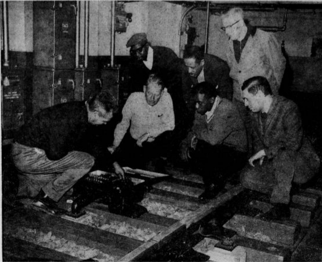
SIGNALS — William F. Eller, left, a signal maintainer, explains the working of a safety device for stopping a train automatically in the event it passes a danger signal. He is working on a 100-foot length of track, complete with ballast, ties, switches and signals, which occupies a part of the school.
